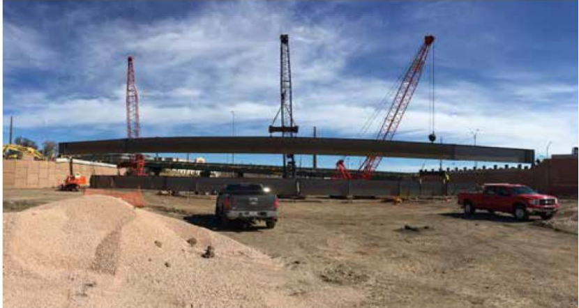
Steel bridge girders have started to be delivered, bolted together and set into place on the bridge pilings. A total of 12 girders will be installed and concrete bridge deck placement will begin following girder installation.
