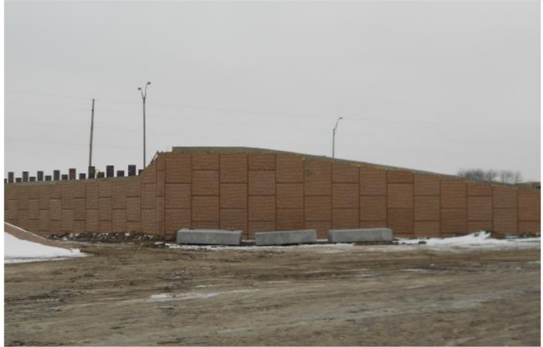
A Mechanically Stabilized Wall on the south bridge abutment is being installed. At it's tallest point, this wall is approximately 25 feet high. A similar wall is being constructed on the north side.
