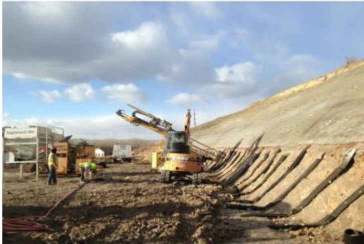
Five rows of soil nails were installed, which included 205 nails (8,410 linear feet of nail). The slope is further stabilized by two inches of flashcoat and four inches of reinforced shotcrete face to prevent sloughing.
