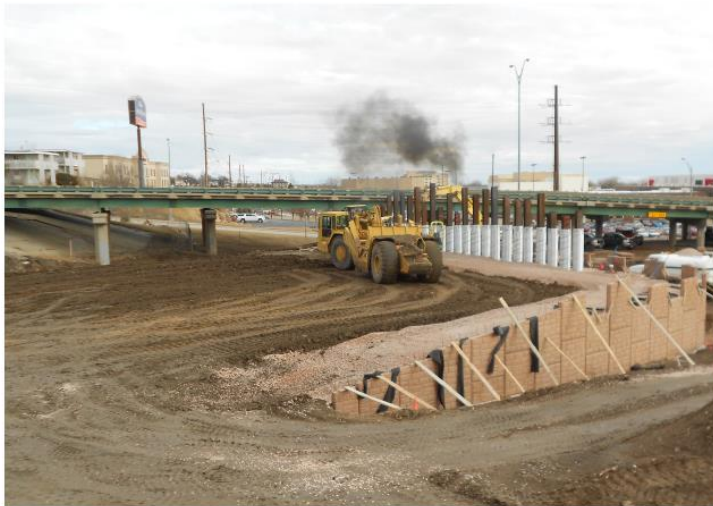
Mechanically Stabilized Walls on the south and north bridge abutments are being installed. At their tallest point, the walls will be approximately 25 feet high.
